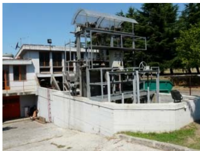
Inlet screens and screw pump
