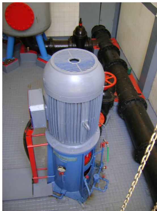
Recent Zagoric Installation
